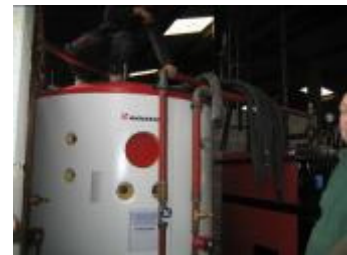
Buffer tank holds a reservoir of 4000 litres of hot water
